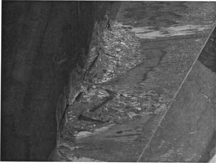
Figure 3.31. Photograph of the damage to Beam 1 in the Osceola bridge.
