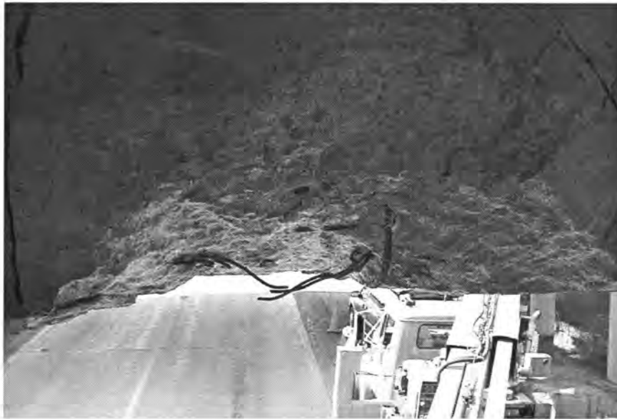
Figure 3.40. Photograph of severed prestressing strand on Beam 9 in the De Soto bridge.
