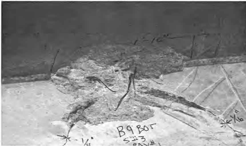
Figure 3.41. Photograph of severed prestressing strand in the De Soto bridge.
