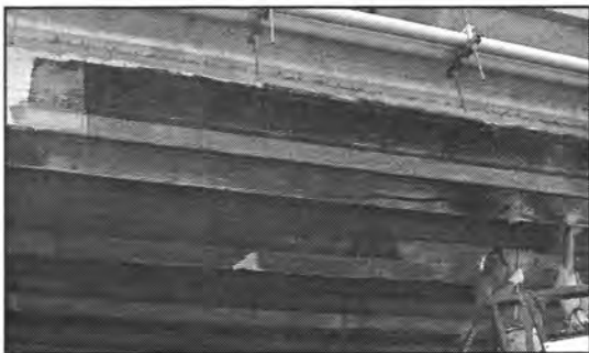
Figure A20. Entire beam after the longitudinal and transverse FRP are installed.
