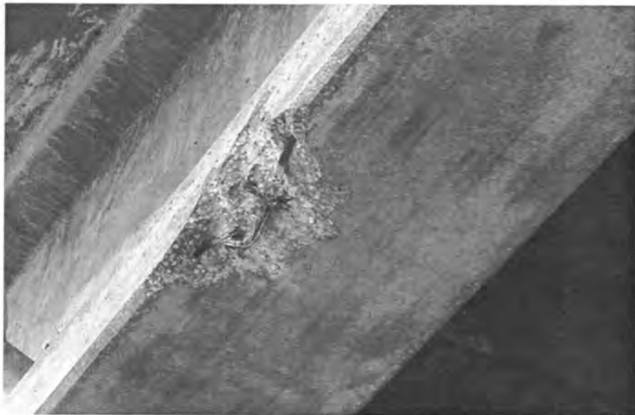
Figure 3.20. Photograph of the damage to Beam 1 in the Altoona Bridge.
