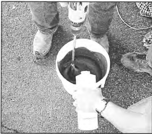
Figure A11. Mixing the blue and color-less component of the saturant layer.
