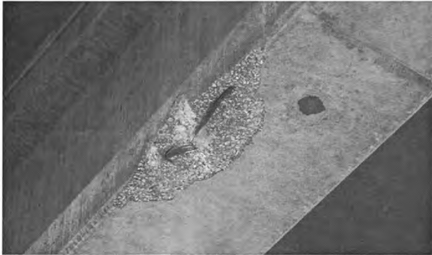
Figure 3.21. Photograph of the damage to Beam 5 in the Altoona Bridge.
